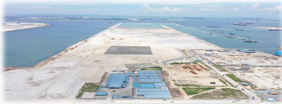
Penta-Ocean / Hyundai / Boskalis Joint-Venture Tuas Terminal Reclamation, Wharf Construction and Dredging Phase 2 (TTP2) Project (Japan, S. Korea, The Netherlands, Singapore)
